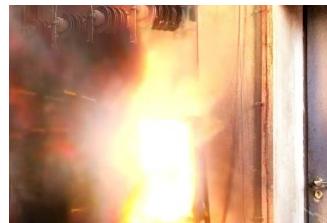
High Power DC Testing
